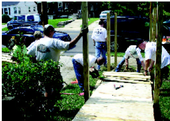
International Paper employees repaired a ramp walkway for people with special needs as part of United Way's Day of Caring kickoff service event in September, 2008.
